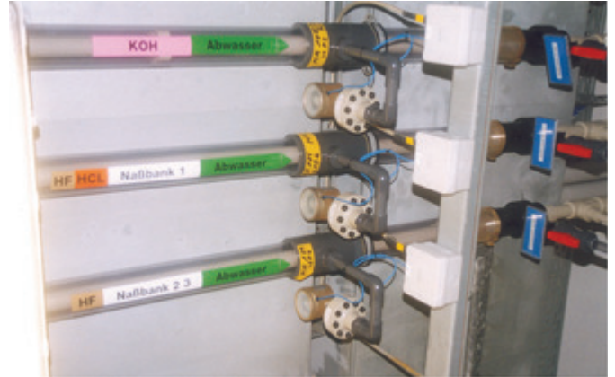
Drainage system für HCl, HF and hydrocarbons in the semiconductor industry
