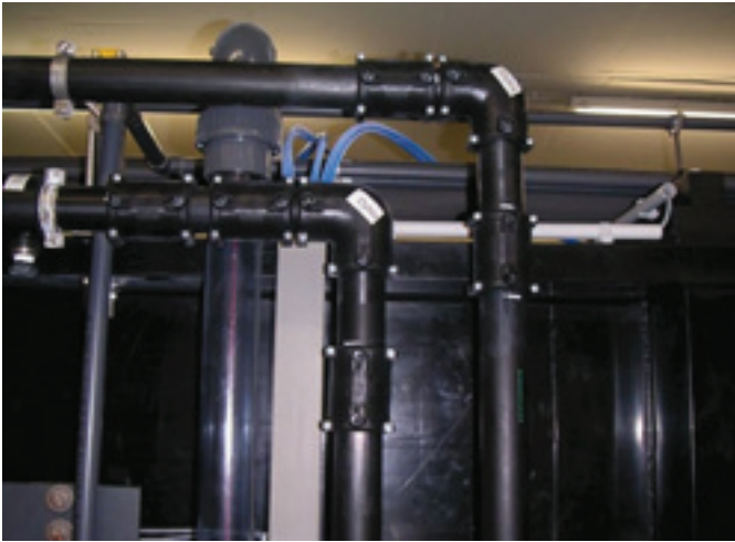
Hydrochloric acid and caustic soda solution for water treatment
